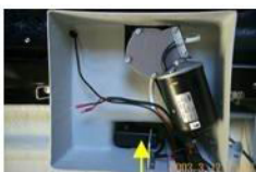
Battery Charger in dome rotation motor box
