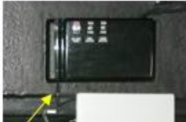
Galib connecting 2 motorbatteries for re-charging
