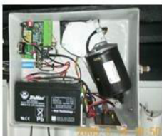
Dome rotation motor box with MaxDome installed
