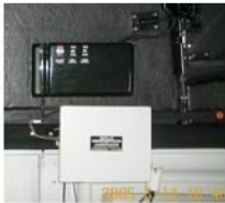
Dome and shutter motor boxes
